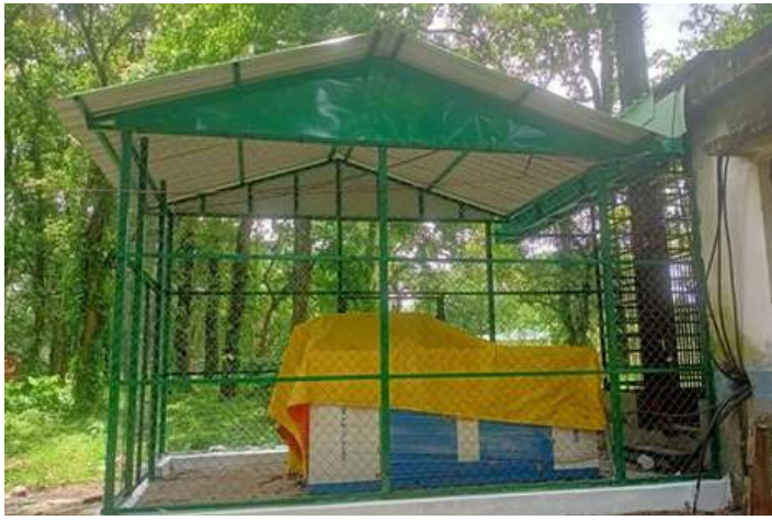
New generator house
